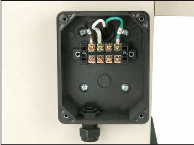
Figure 123. Power junction box wiring.
